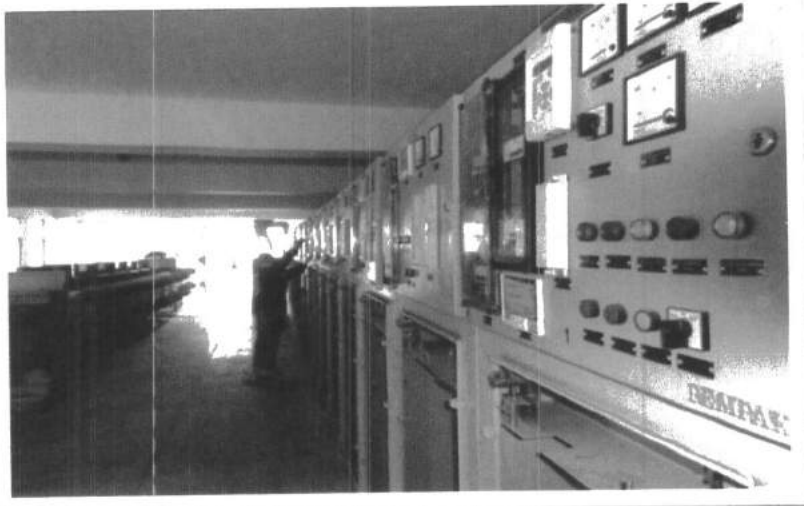
Wana Grid Station.
